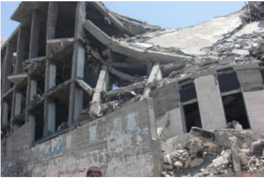
Unsafe building, Gaza city
