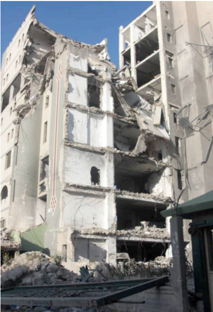
Remains of large apartment block
