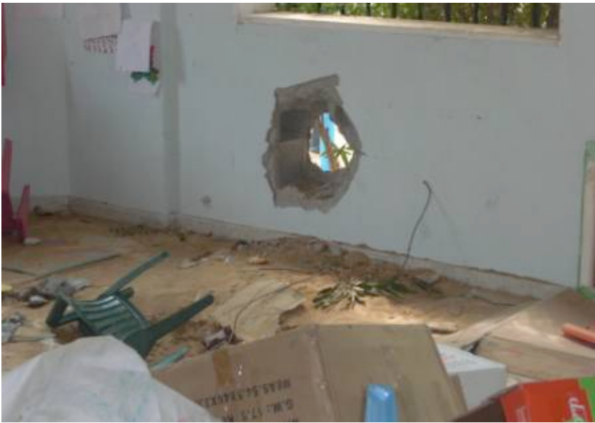
Classroom damaged by rocket attack
