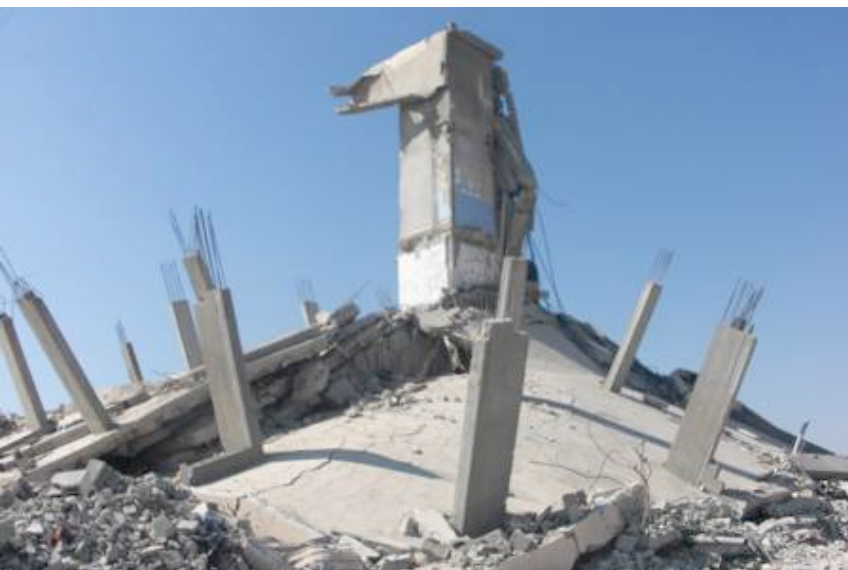
Bombed home near the industrial area
