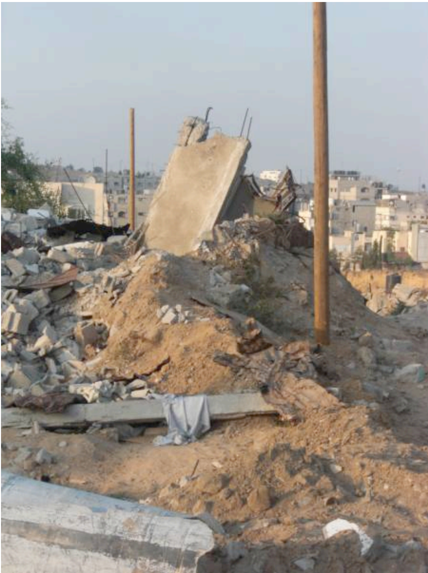
Former home reduced to rubble
